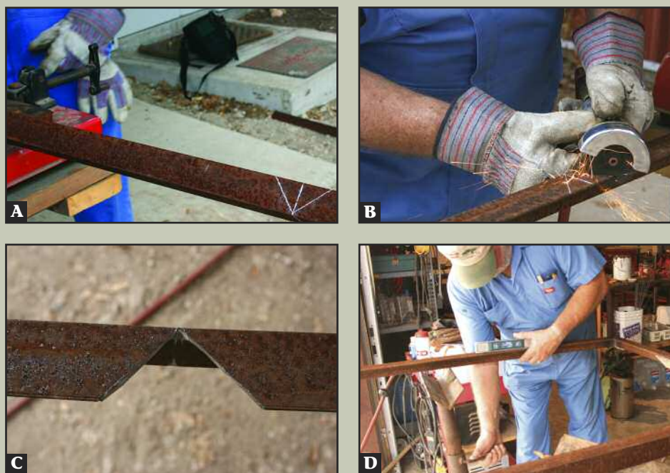
A piece of angle iron marked for cutting (A). After cutting (B and C), the iron can be heated and bent to form the desired configuration (D). The bracket is then welded. Designs may differ, depending on the door style.
